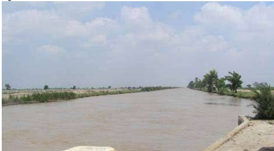
Figure 3.2: Eroded berms on the Mithrao Canal
